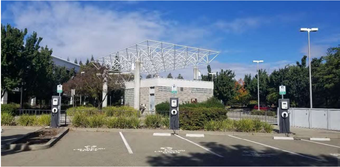
Figure 26. San Ramon Transit Center EV Charging Stations
