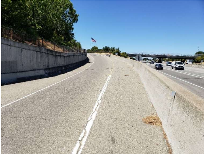
Figure 4-19 Retaining Wall at the Alcosta Boulevard On-Ramp Approaching the Merge with the San Ramon Valley Boulevard On-Ramp
