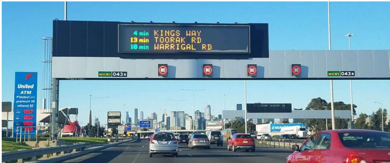
Figure 1-2 Managed Freeway Installation on M-1 Monash Freeway, Melbourne, Australia
