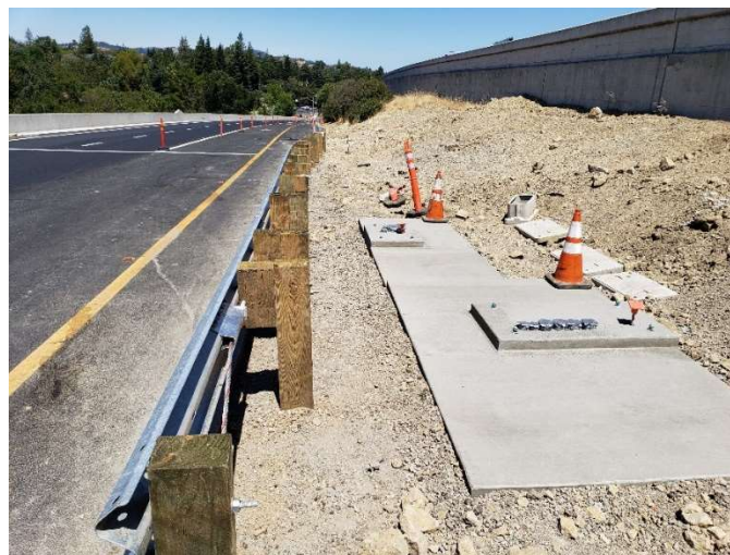
Figure 4-16 ITS Installations at the Reconstructed Rudgear Road On-Ramp
