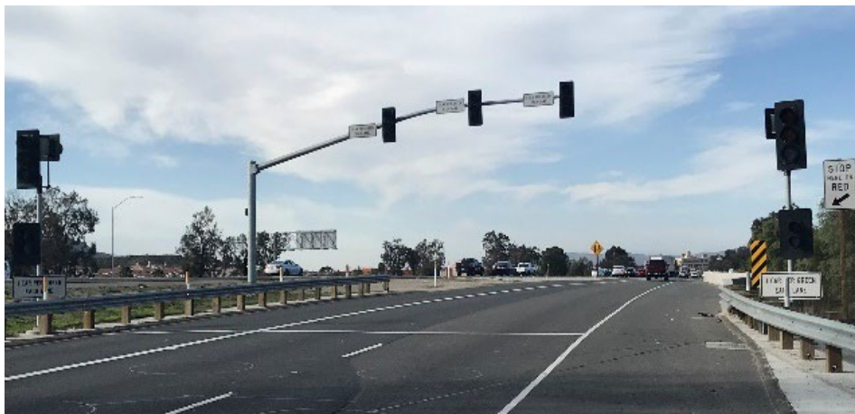
Figure 7-5 Typical Ramp Meter Signals
