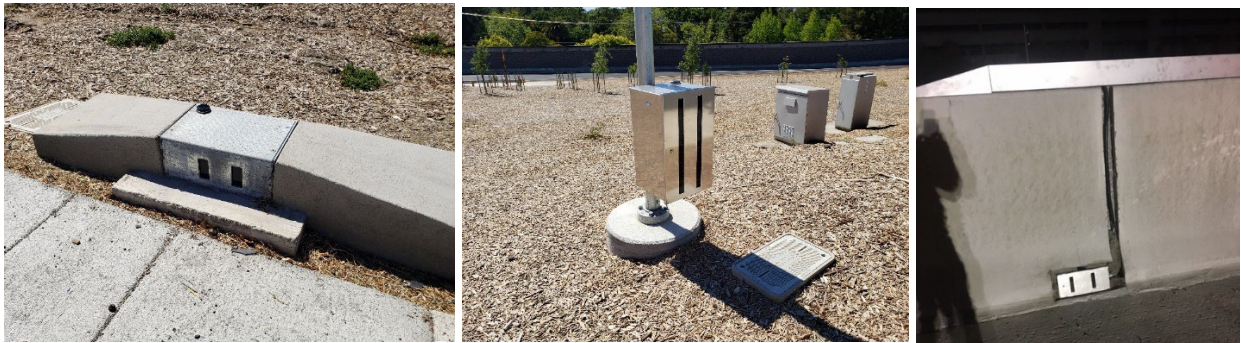
Figure 7-8 Typical TIRTL Installations
